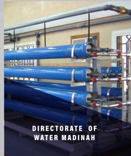
Reverse Osmosis Plant At Wadi Al Fara
